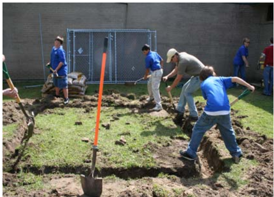
Middle school students help LSU Coastal Roots staff dig the trench for the irrigation system.
